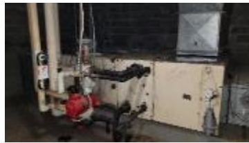
Air Handling Unit
