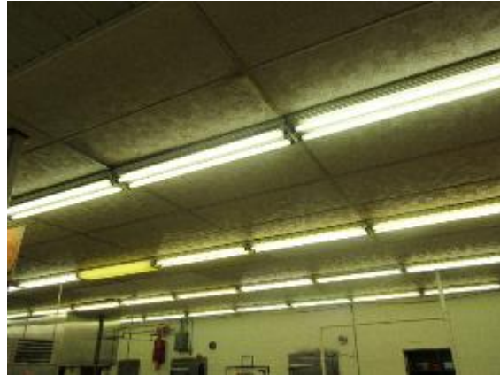
Macopin Middle School Lighting
