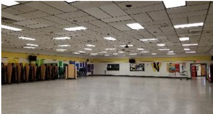
West Milford High School Light Fixtures
