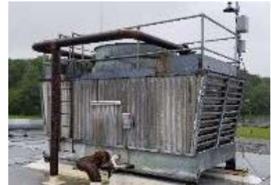
High School Cooling Tower
