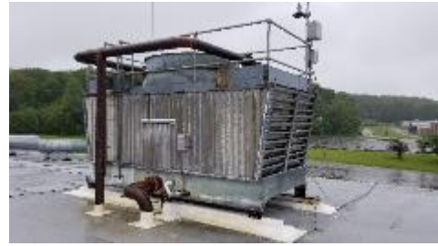
Chiller Water (CHW) Cooling Tower
