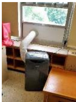
Portable HVAC Unit
