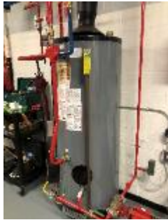
Domestic Hot Water
