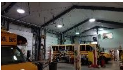
Bus Garage Lighting
