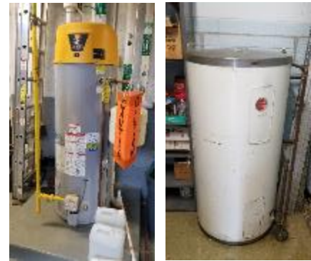
Domestic Hot Water
