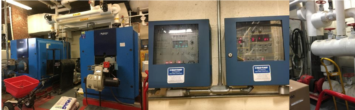
Figure 11 – Hot Water Heating System
