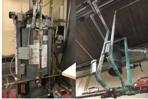
Figure 15 – Domestic Hot Water System and Missing Pipe Insulation
