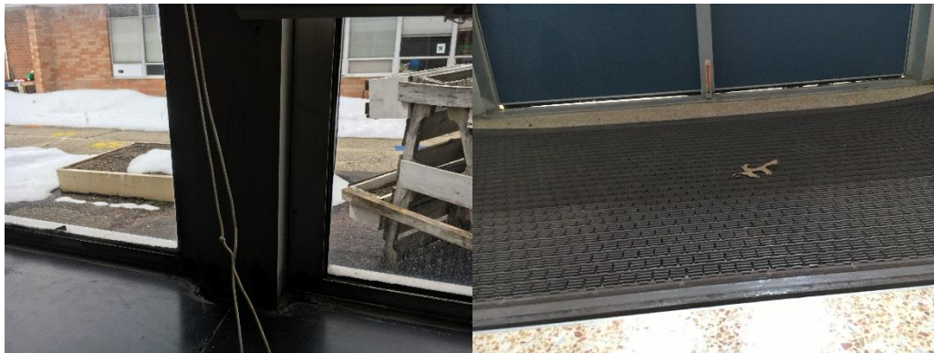
Figure 7 – Building Envelope Deficiencies
