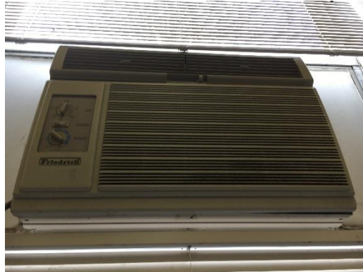
Figure 13 – Typical Window AC Unit
