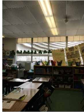
Figure 9 – Lighting Fixtures in Poor Condition
